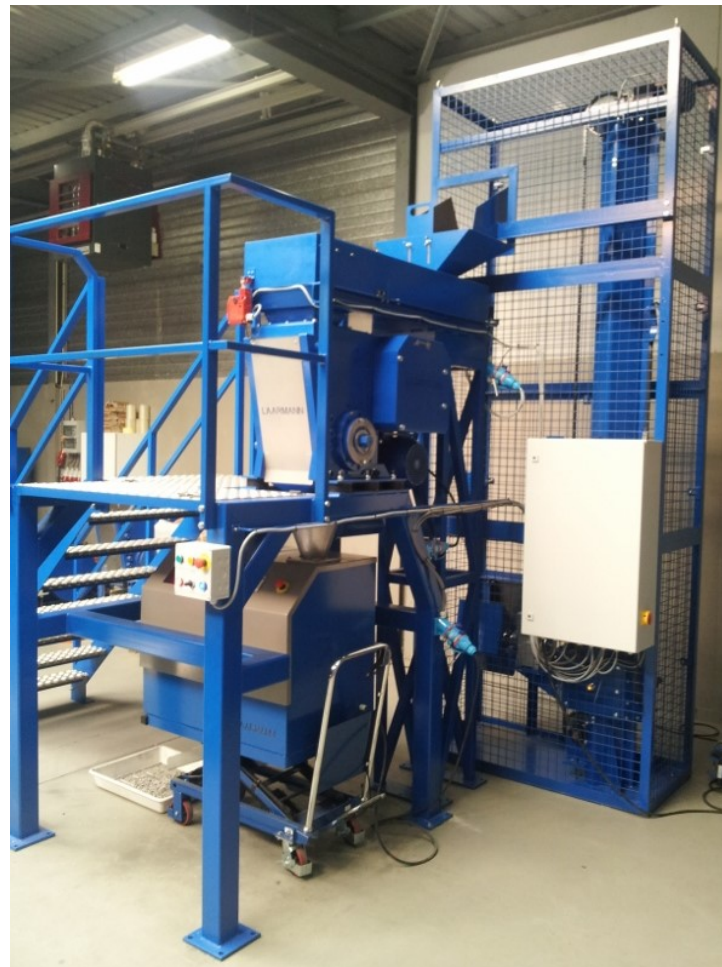
Crushing installation with LMFC250 fine crusher and rotary sample divider
